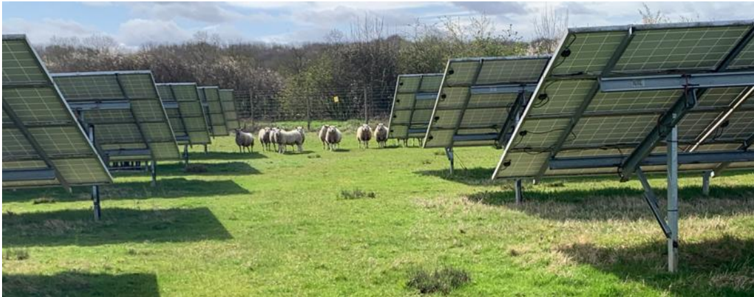
Photo 39: Grass growth below and between arrays
