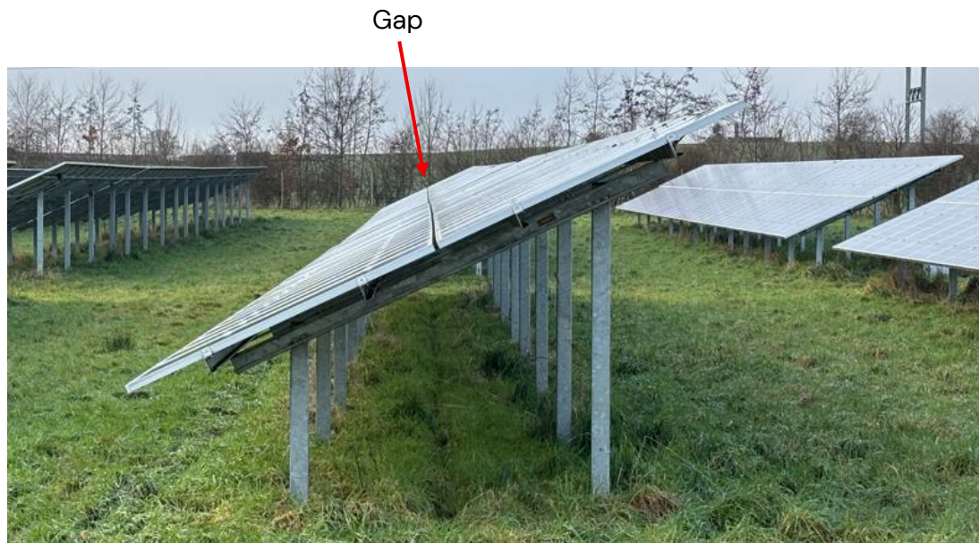
Photo 38: Panels array showing gaps between panels and between rows of panels
