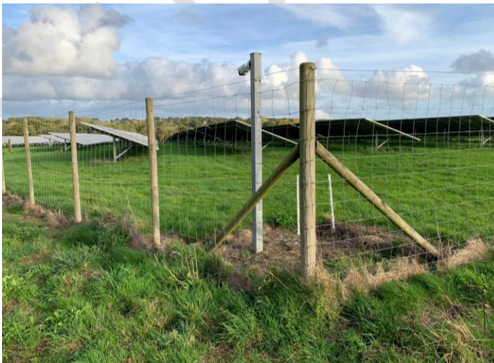
Photos 50 and 51: CCTV Poles and Fencing
